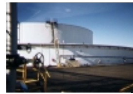
Managing Above-ground Storage Tanks releases can be a challenge.
