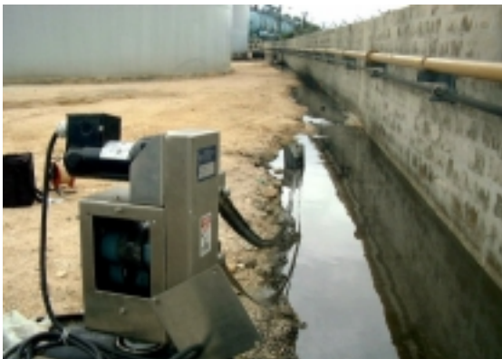
At a site in the Caribbean, the NTST series NET system was adapted to recover a surface spill of petroleum products within an above ground storage tank farm.
